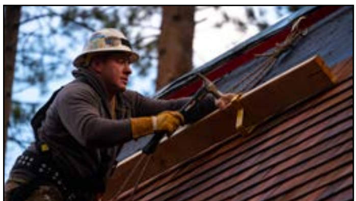
U.S. Air Force Master Sgt. Dominic Tanzi, 152nd Civil Engineer Squadron operations management noncommissioned officer in charge, hammers a nail into a support beam at the Tallac Historical Site, South Lake Tahoe, Calif., October 21, 2021. Tanzi has been training and working on projects with the U.S. Forest Service at the Tallac Site since he joined the unit in 1998. (U.S. Air National Guard photo by Airman 1st Class Thomas Cox)
